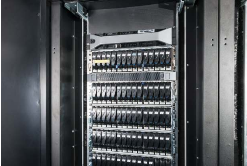
Figure 11.14 A storage array.
